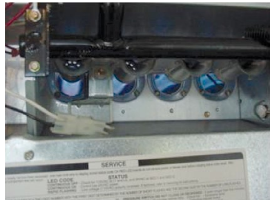
Light blue flames indicate clean efficient combustion.
