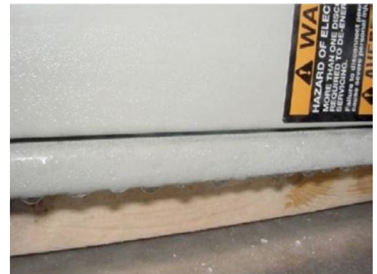
Condensation at bottom of air handler caused by wet interior insulation, rendering the insulation useless.
