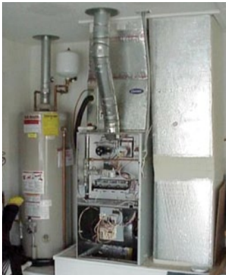
Gas furnace with panel removed. Cabinet and return duct leakage can interfere with natural draft appliances such as the gas water heater at left.
