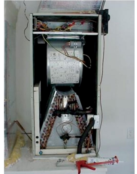
Inside view of AHU with blower above evaporator coil. Electric heat element is located above the blower.
