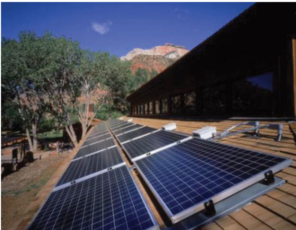
Crystalline modules mounted on a sloped roof. Source: Florida Solar Energy Center
