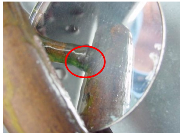
Mirror and dye used to locate leak.
